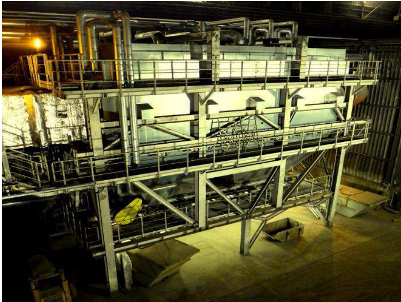
Overview of Waste Heat Boiler
