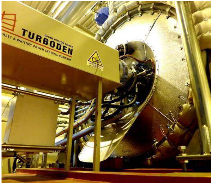
Turboden unit installed
